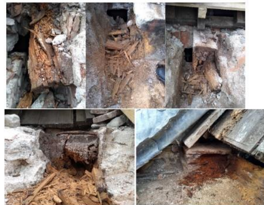
Figure 5. Typical condition in which the timber ties were found when inspected from the exterior side of the roof. In these images, not all decayed wood had yet been removed from the elements.
