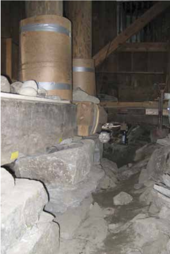
New foundations under the raft beams, work done during the Stave Church Preservation Programme. Photo: Marit Westli Arntzen 2009.
