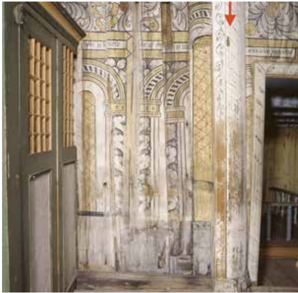
Intermediate post in the north wall of the chancel, marked with a red arrow. Damaged above the ceiling and under the floor. Photo: Birger Lindstad and Joppe Christensen 1995.
