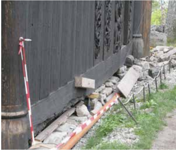
Rot-damaged sill beam on the north wall of the nave. The foundations were repaired, but not the rotten material, as it is not load-bearing. Photo, Sjur Mehlum 2009.
