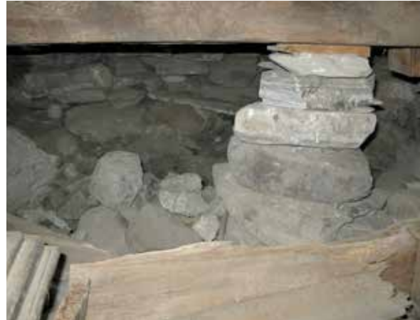
Unsteady, incomplete foundations under the raft beams, put in place around 1970. Photo: Ina Borgen Snarud 2008.
