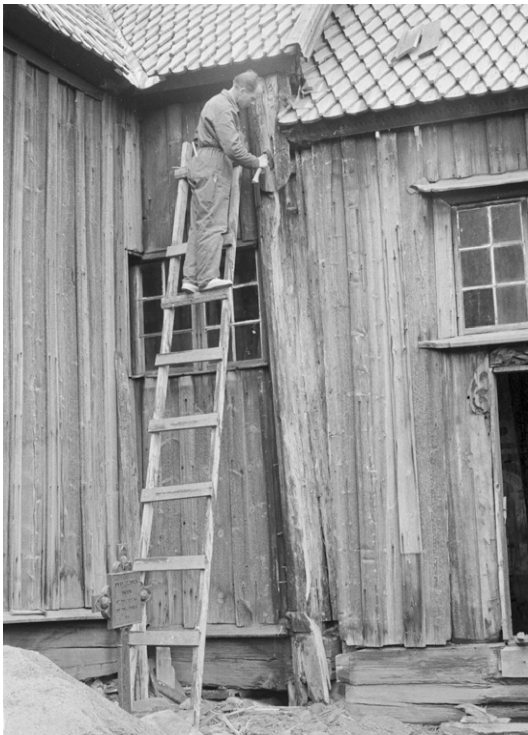
Nore Stave Church. South-east corner post of the nave has extensive rot damage along the whole length of the post. It was also repaired in 1969. Photo: Arne Madsen 1969.
