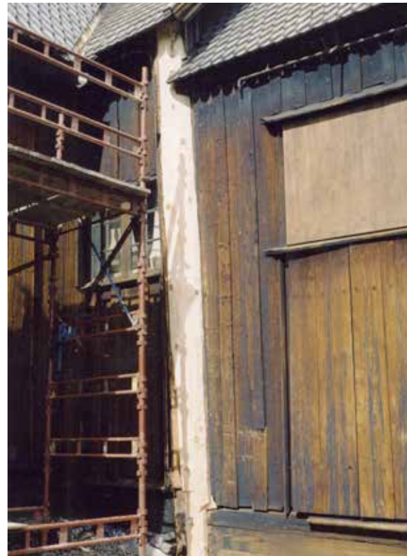
Repaired south-eastern corner post. The post was then panelled as it was before repair work commenced. Photo: Hans Marumsrud 2003.
