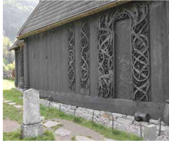
New foundations under the sill beam on the north wall. The sill has been raised by about 10 cm with good clearance from the ground. This will help prevent further rot damage. Photo: Leif Anker 2013.
