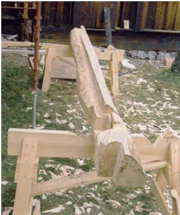
New, adjusted post for repairing the south-east corner post. The west side of the post is adjusted to the rot damage. This method secured the support of the roof while preserving the interior of the church. Photo: Hans Marumsrud 2003.
