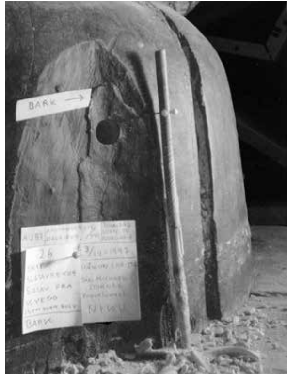
Ill. 23. Stave in Kaupanger stave church with damage. Photo: Jan Michael Stormes 1998.
