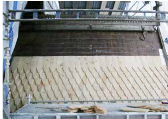
Replacing roof shingles at Hopperstad. Unlike Borgund, here the shingles were changed in whole areas. There is no cardboard, foil or other waterproofing beneath the shingles here either. Photo: Nedre Jølster bilelag, undated.
