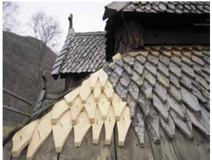
Replacing roof shingles; each shingle was fitted individually. Usable shingles were kept. There is no cardboard, foil or other waterproofing beneath the shingles. Photo: Harald Ibenholt 2009.
