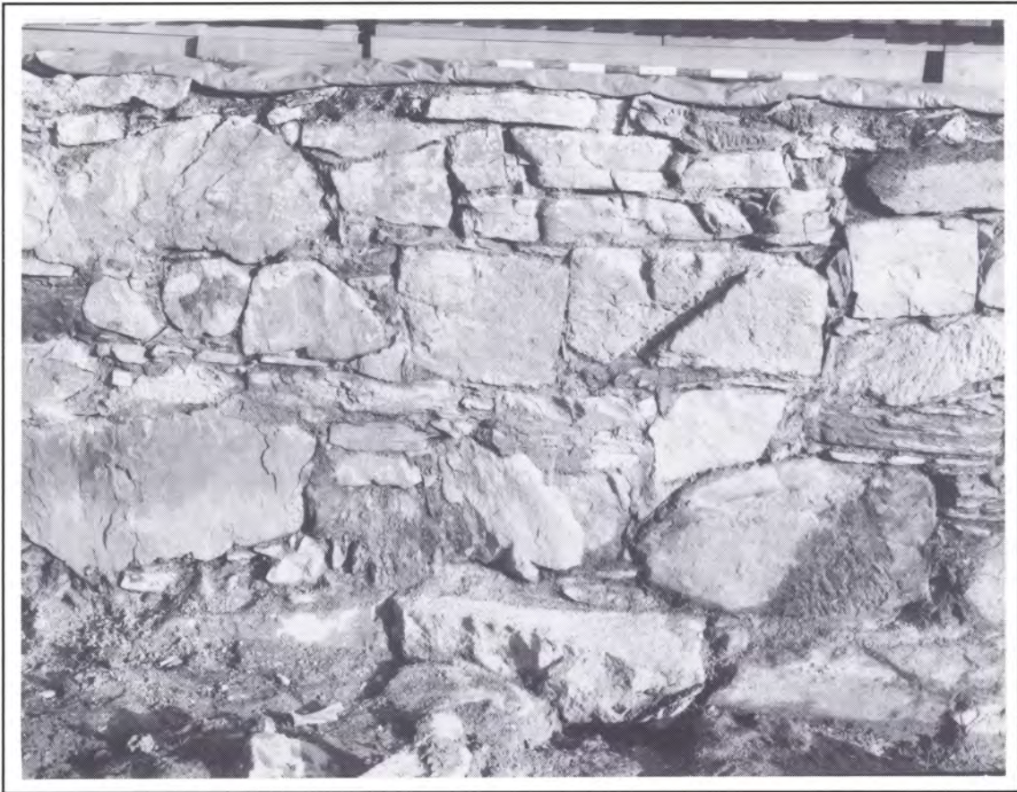
Fig. 10 Curtain wall AK2=BK1: detail of west facing showing oblique slot (cf. fig. 9).
