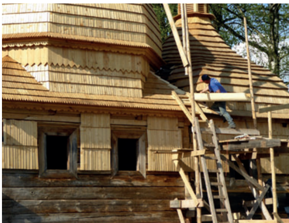
Renovation work at the Nowe Brusno Tserkva, photo by G. Ciećka, private archive
