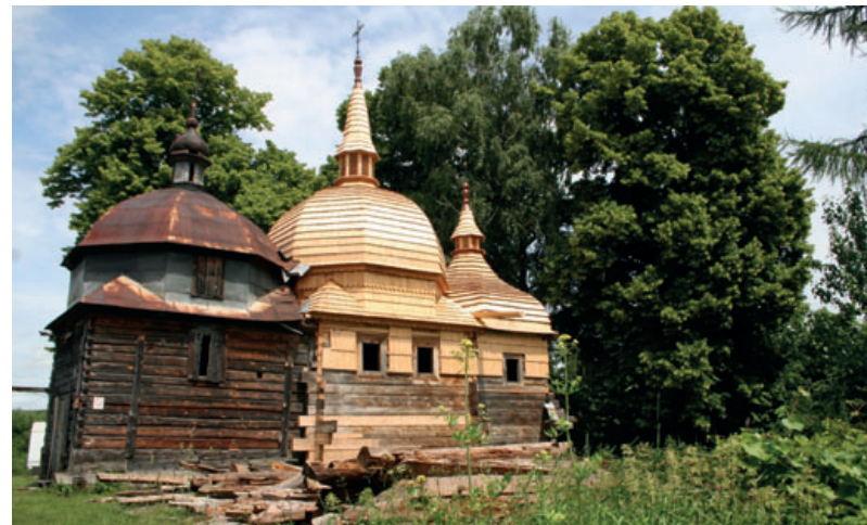
The Tserkva in Nowe Brusno in the course of renovation and conservation work, photo by G. Ciećka, private archive
