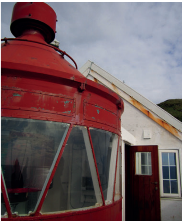
Lantern room of the Kråkenes lighthouse, photo by A. Koziol, private archive
