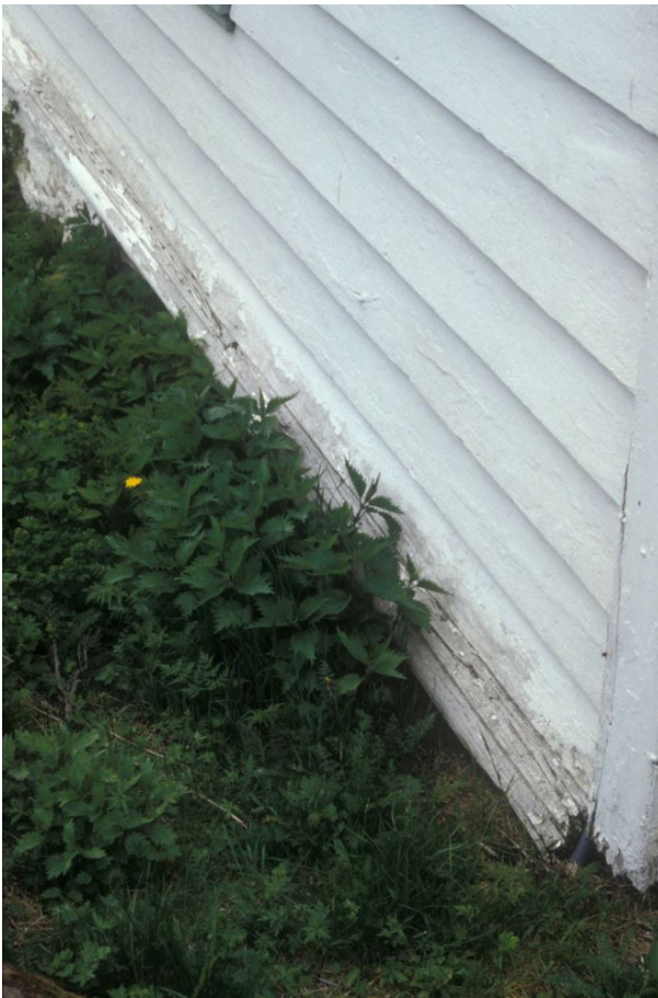
Figure 7.13 Grass growing along wooden walls accumulates moisture and leads to decay.
