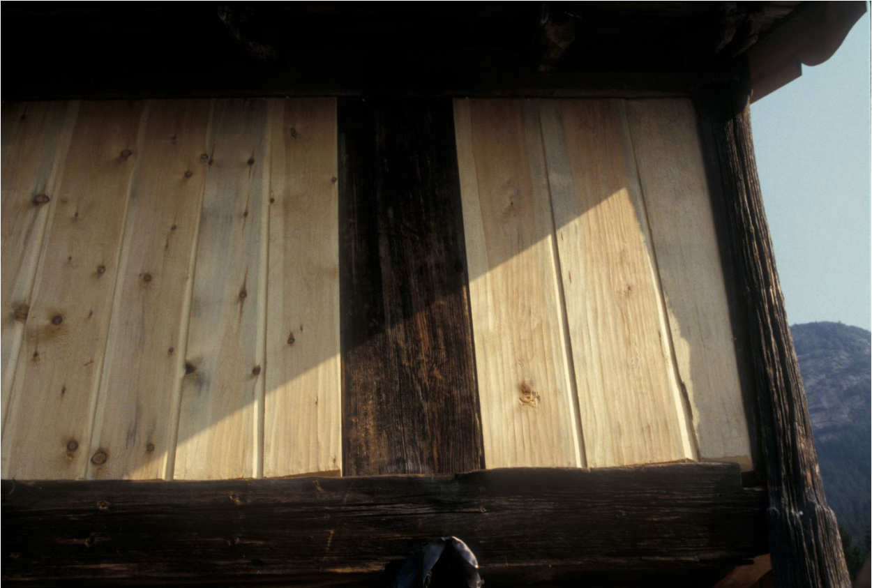
Figure 5.6 Boards inserted into the gallery wall of a Norwegian medieval timber structure during repair work. The boards have been planed using a spokeshave.
