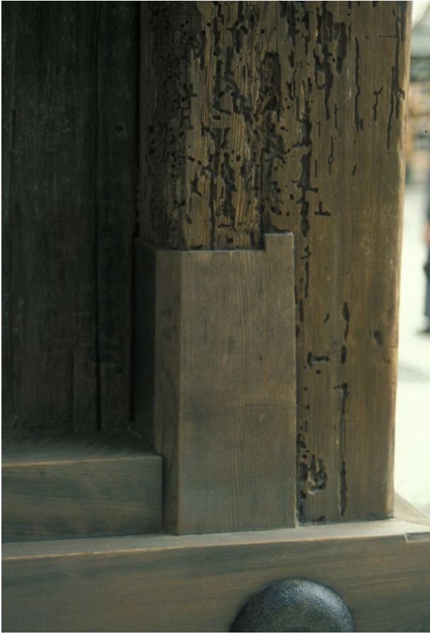
Figure 8.11 Detail of the Shakadō hall in the Kiyomizu-dera Buddhist temple, Kyoto, Japan, built in the eighteenth century. During the dismantling-repair process completed in 1975 the lower part of this corner pillar was repaired by jointing in new, well-seasoned timber. The new timber contrasts dramatically with the original timber, whose appearance is due to decay, insect attack and the effects of weathering.
