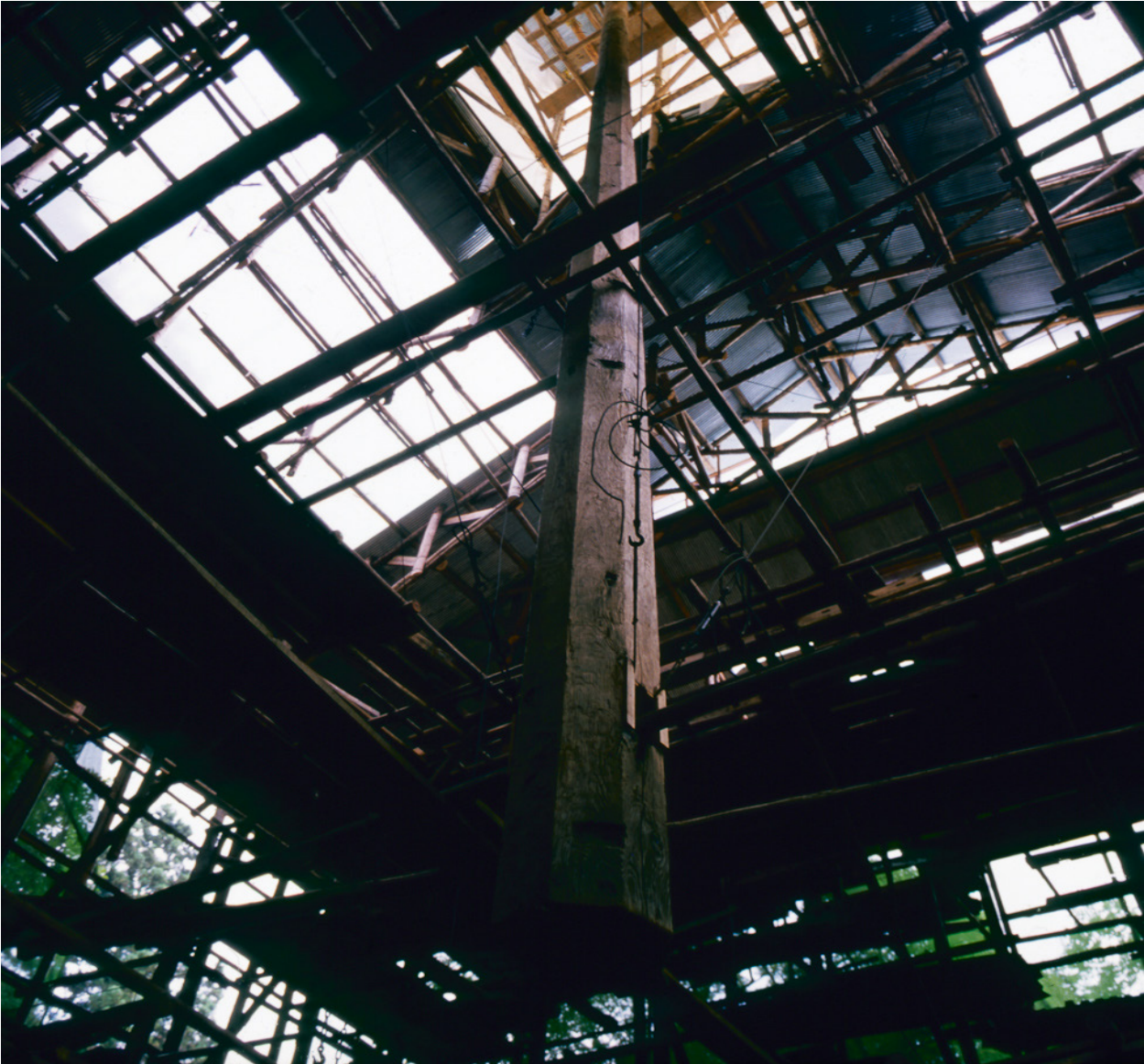
Figure 4.5 The central pillar of the three-storied Oyama-dera pagoda during preservation work in 1989. All members of the pagoda have been dismantled except the central pillar which is suspended from the scaffolding.
