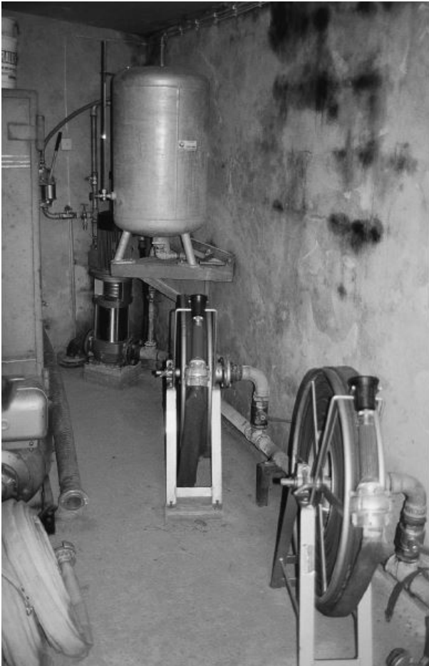
Figure 7.14 Fire protection equipment at a Norwegian farm where there are a number of listed buildings. The owner has created a small pond to provide water for the fire fighting equipment.
