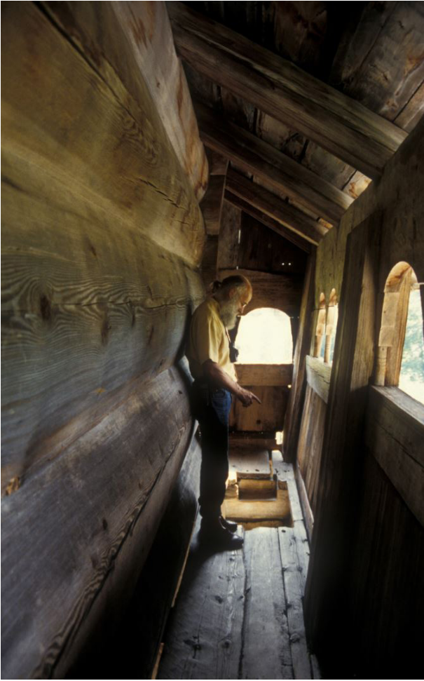
Figure 6.1 Large dimension timber from a late sixteenth century log-structure in Setesdal, Norway.
