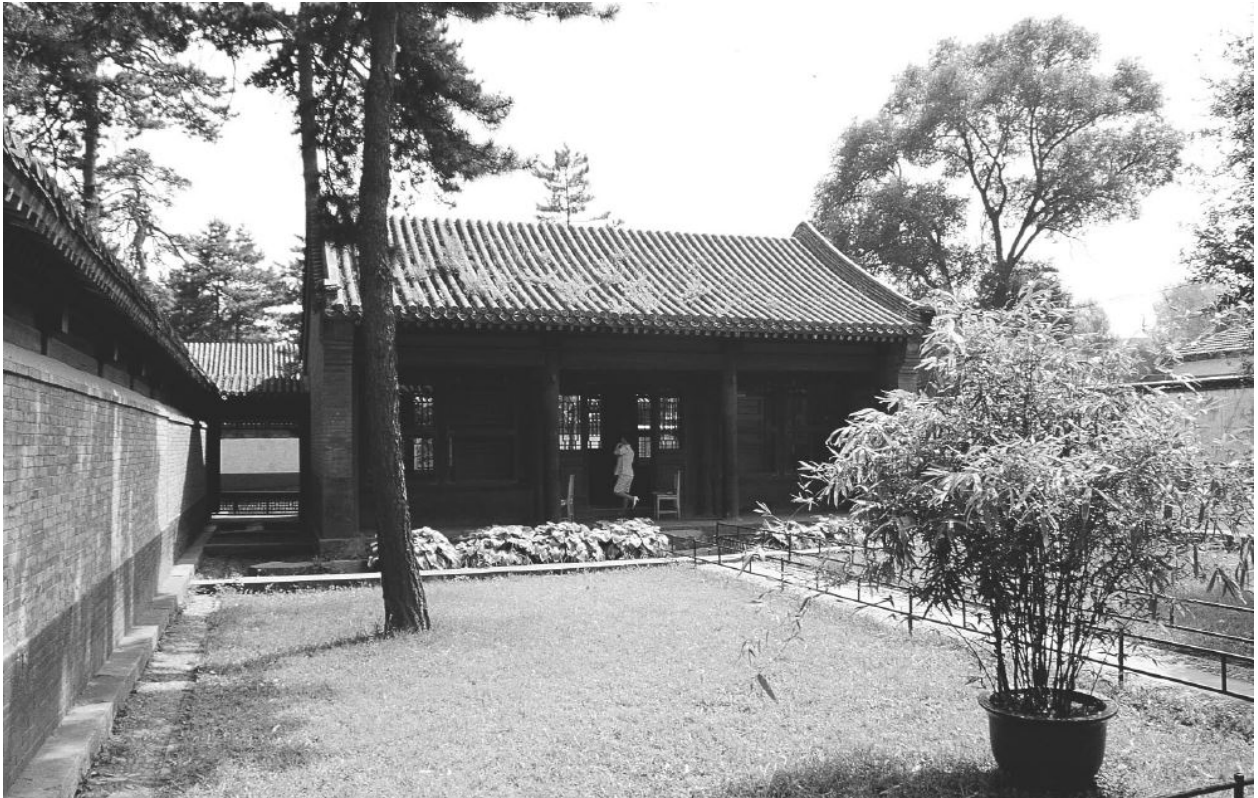
Figure 7.11 The Mountain Resort, Chengde, China, a World Heritage site. Small trees are growing on the roof of the building in the background. It is a part of the site management plan to remove growth from the roofs every three years. The removal is necessary for the long-term protection of the roof timber structure and tile roofing. The roof in this picture had been cleaned one year previously.
