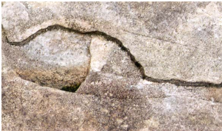
Figure 58. To insulate damage edges and prevent further cracking and flaking, it is common to caulk crack edges with cement. Photo: L. Sæbø.
