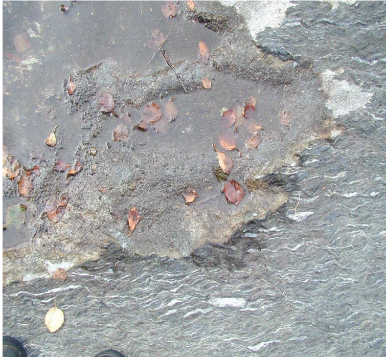
Figure 57. Damage edges with active weathering that have been sealed with cement mortar. Åmøy, Rogaland. Photo: AmS.
