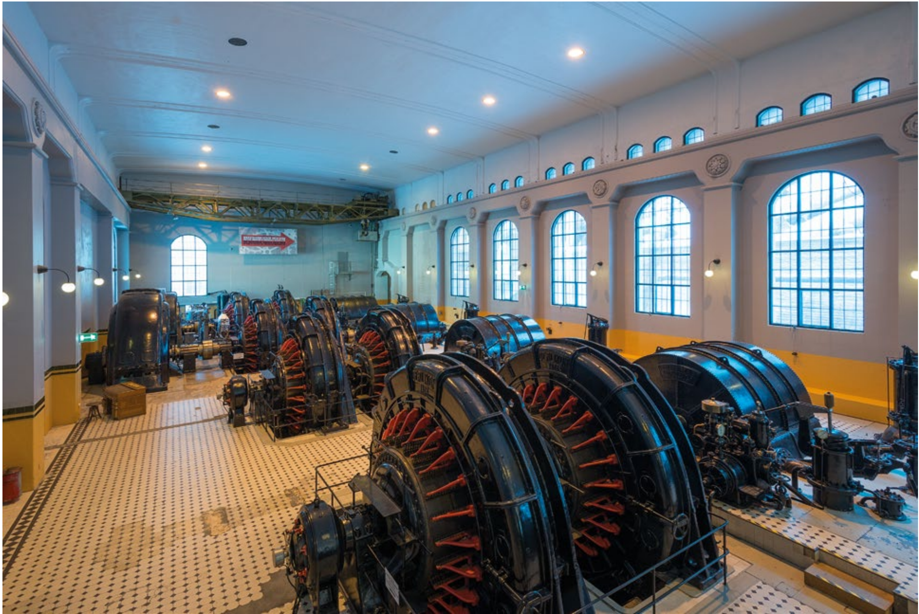
Fig. 25 Vemork Power Plant. Photo: Per Berntsen
