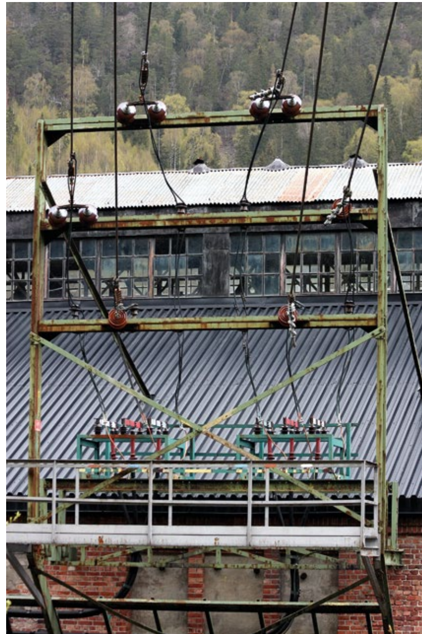
Fig. 37 Power line 16/17. Photo: Eystein M. Andersen
