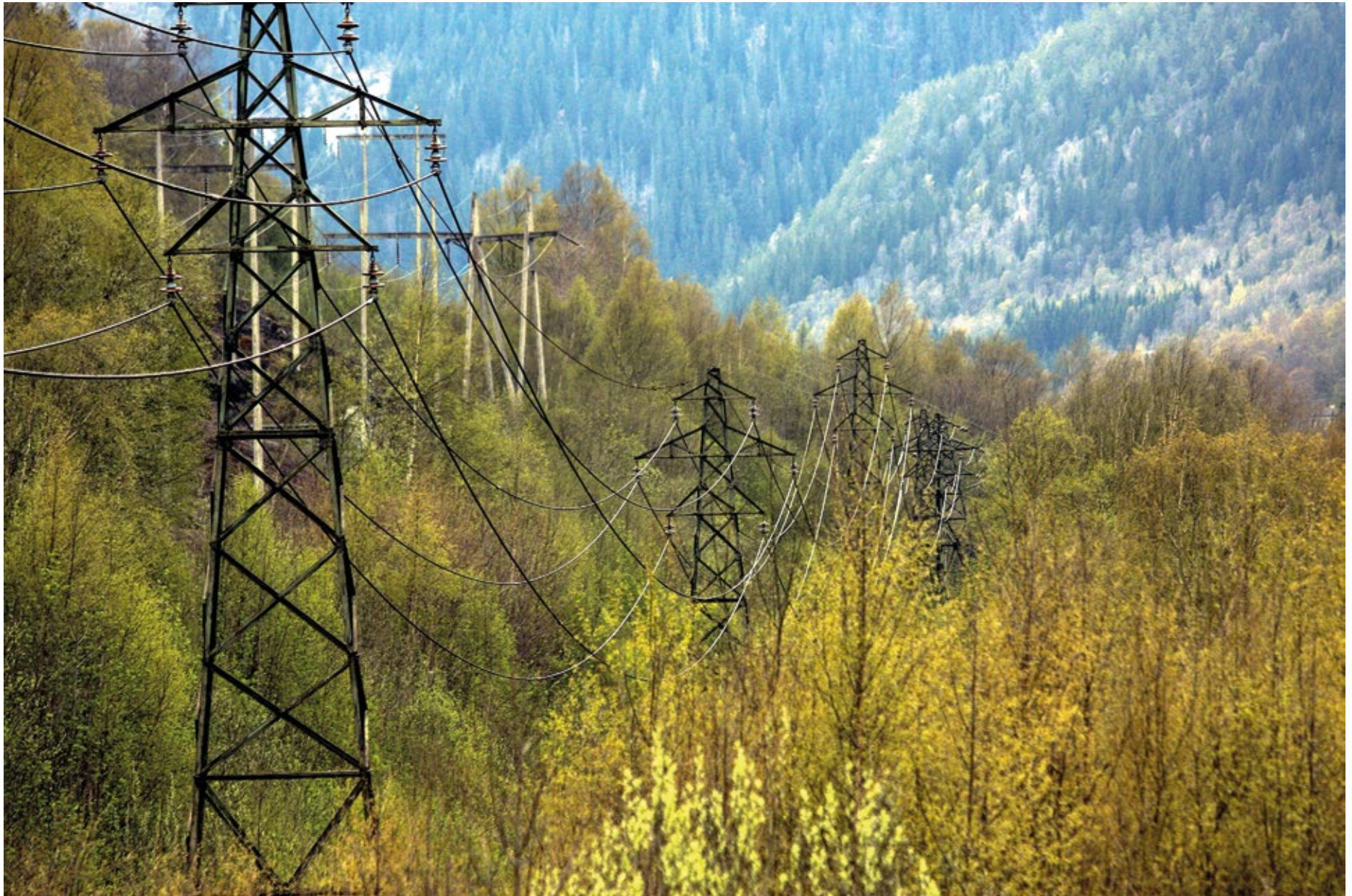
Fig. 36 Power line 16/17. Photo: Eystein M. Andersen
