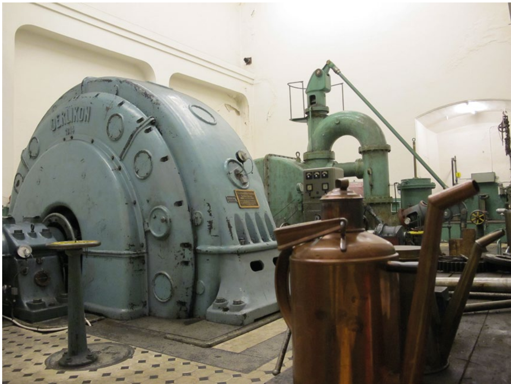
Fig. 35 Såheim Power Plant, underground turbine generator hall. Photo: Trond Taugbøl
