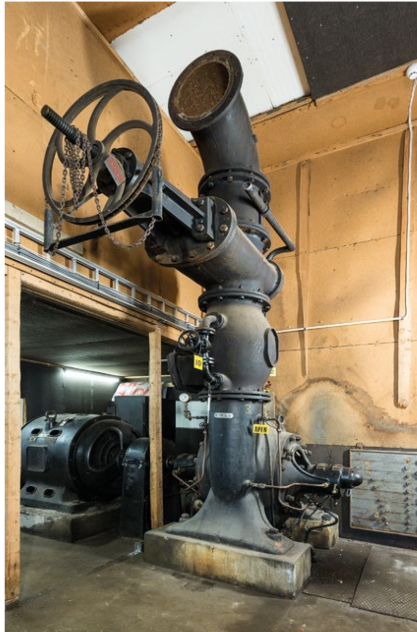
Fig. 62 AEG Pump in Pump House, Hydro Industrial Park in Rjukan. Photo: Per Berntsen
