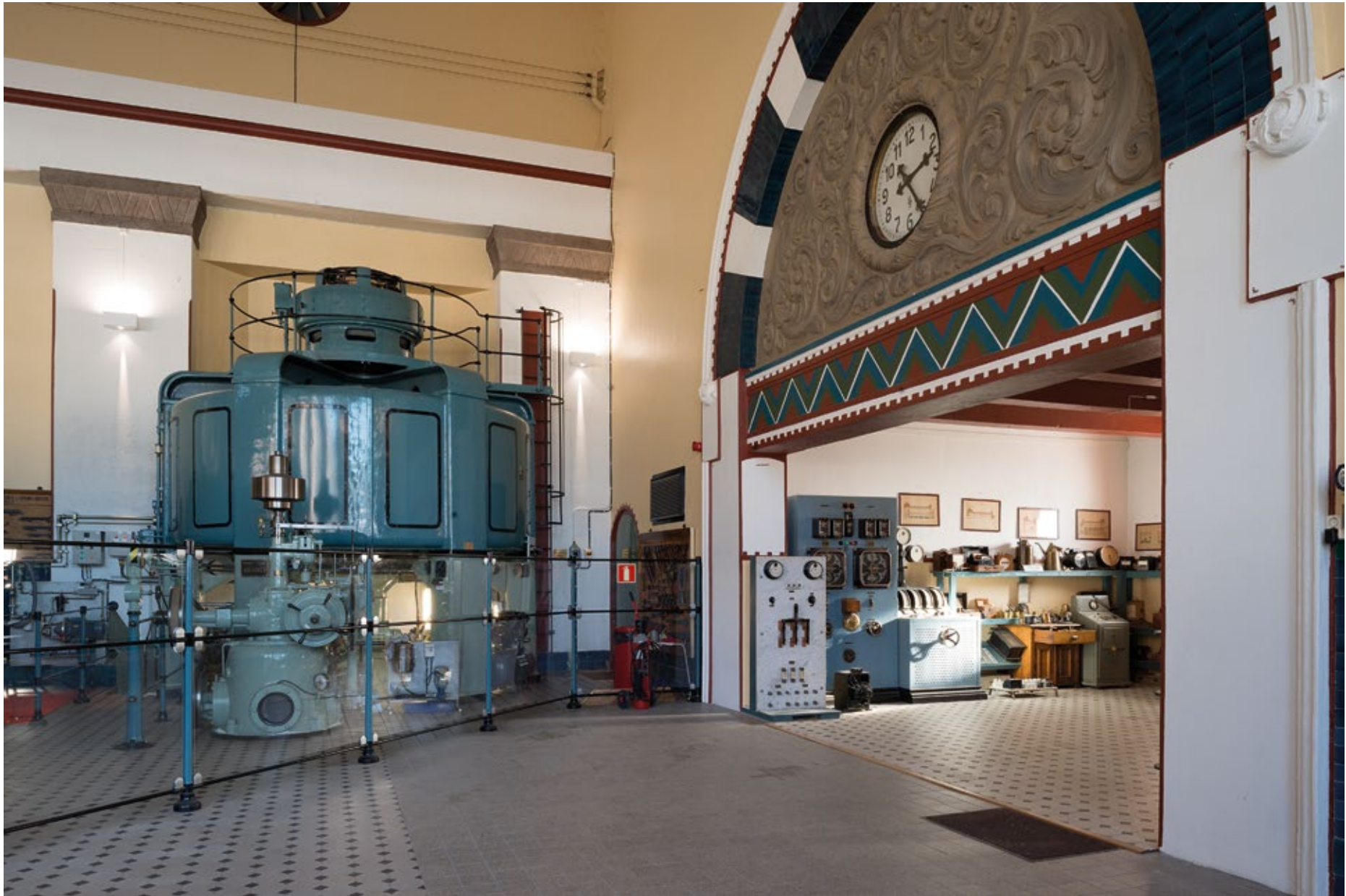
Fig. 13 Tinfos II Power Plant. Photo: Per Berntsen
