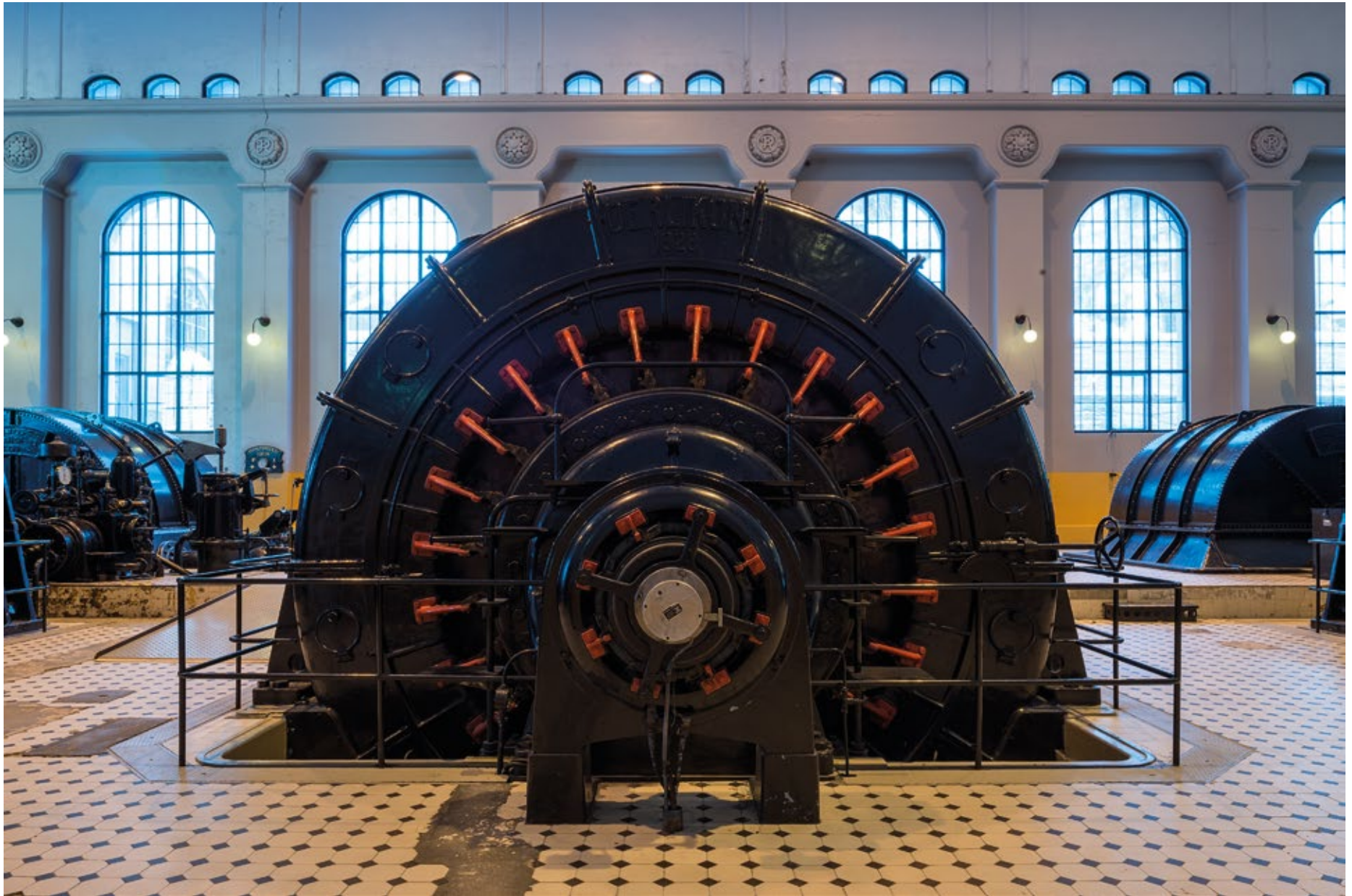
Fig. 26 Vemork Power Plant. Photo: Per Berntsen
