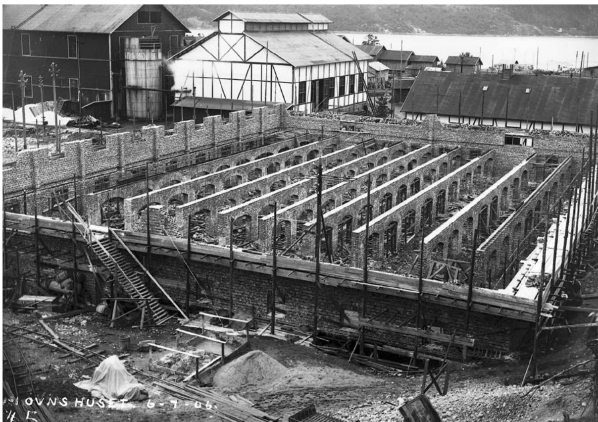
The construction of Furnace House A in June 1906 with the buildings of Hydro's Test Factory behind. Photo: Norwegian Industrial Workers Museum.
