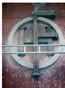
The Rjukan House with the old emblem on the facade was restored back to its original appearance in 2012. Photo: Eystein M. Andersen.
