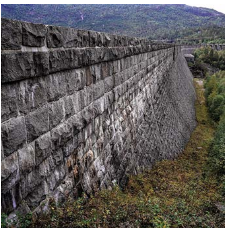
The granite dam Ringedalsdammen raising lake Ringedalsvatn up to 464 m.a.s.l. is part of the Tysso I power plant scheme. Photo: Birger Lindstad.
