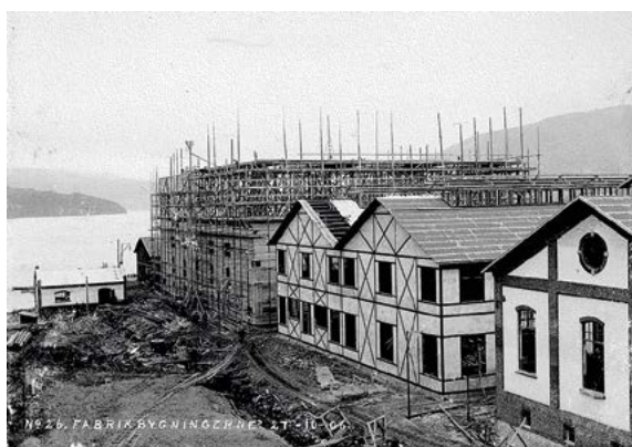
Birkeland's experiments ended in 1905 at Notodden, where a test factory quickly was built. Here the furnace house and the tower house under construction in 1906. Photo: Norsk Hydro
