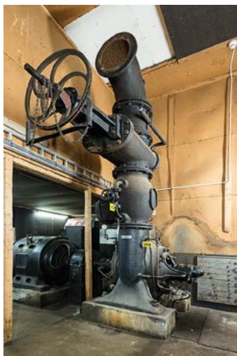
The AEG Pump in the Pump House. Photo: Per Berntsen.
