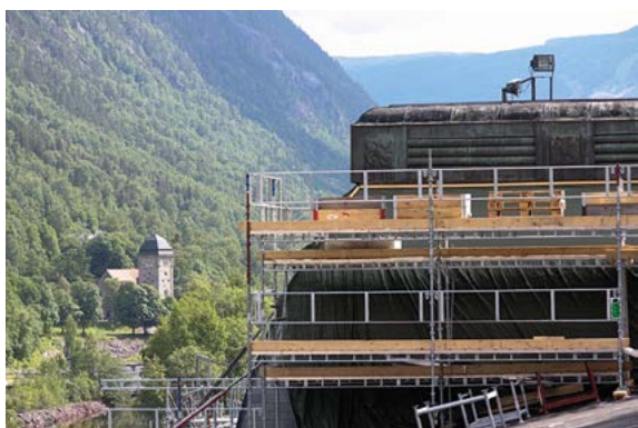
Såheim power station building was under restoration in 2012. Photo: Eystein M. Andersen.
