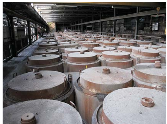
The more than 300 ovens of the Frank-Caro type in the Cyanamide factory are a unique feature at the Odda Smelteverk. Photo: Trond Taugbøl.
