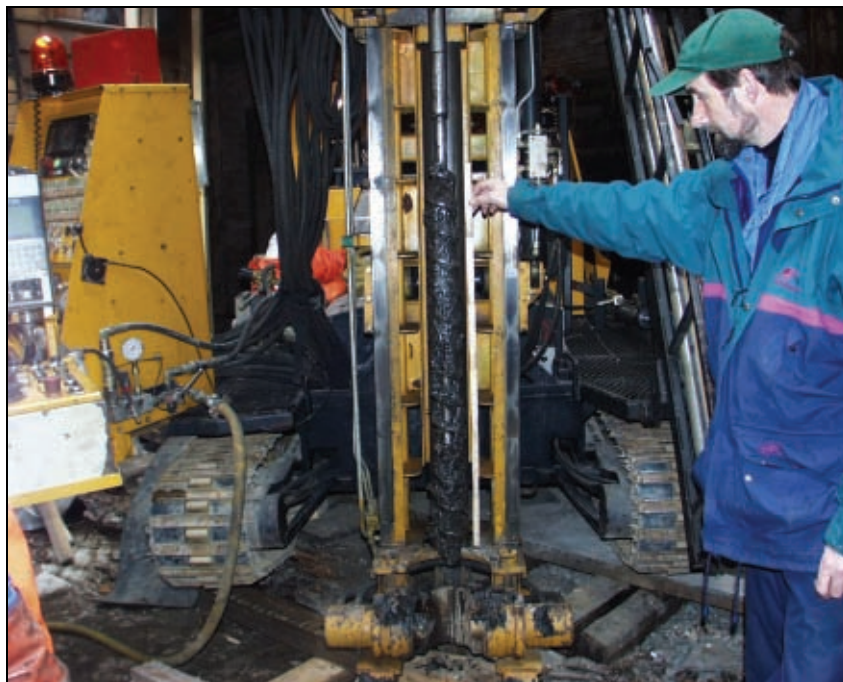
Sampling with 100 mm auger on rig inside building IVe, Svensgården tenement, Bryggen, Bergen (photo: Jensen, Multiconsult AS).
