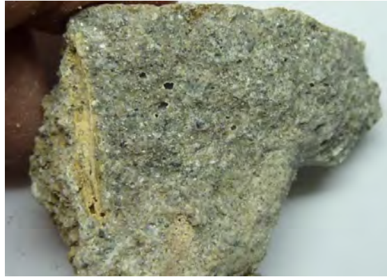
Plate No. 2: Close-up of a section of the pointing mortar with soiling on the outer surface, left side of plate.
