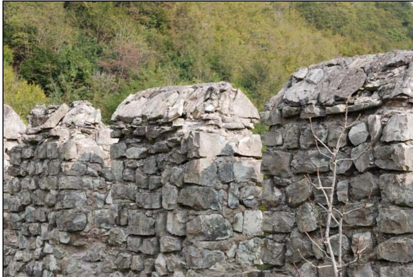
Crumbling cement on the reconstructed toothed 4 th C. defence wall.
