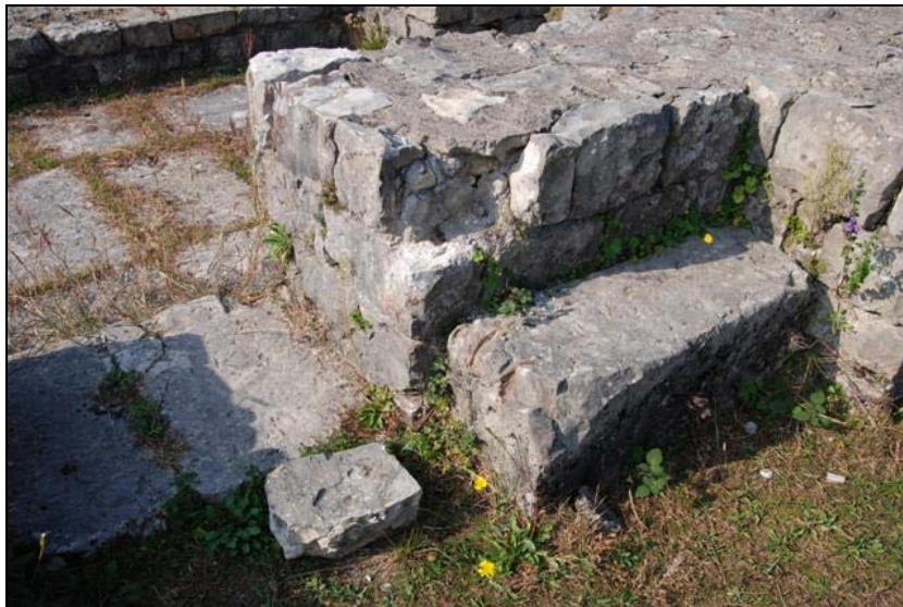
The wall top of part of the Royal Bath: Cracked and crumbling cement. A stone block has fallen out.
